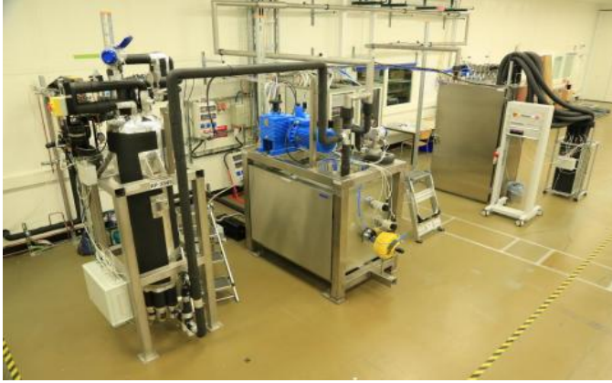
Figure 1: 15kW TIF plant at CERN
